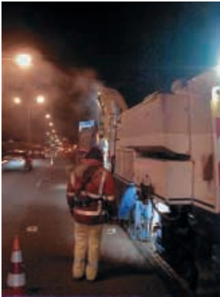
'Workers exposed to hazardous substances'
